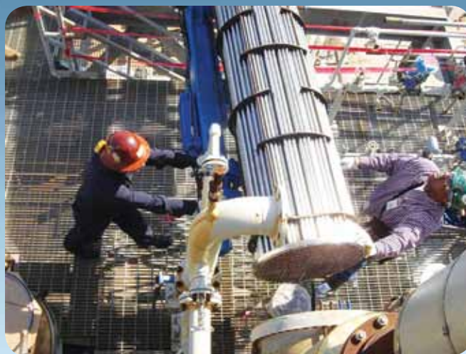
Aerial extractor pushing back an exchanger bundle.
